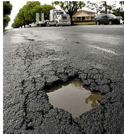
The Warrego Highway has already been damaged by heavy traffic and wet weather.
